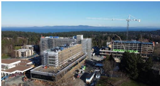
Drone shot of the Dining and Dorms project at UVIC photo from January 2022, off UVIC's website
