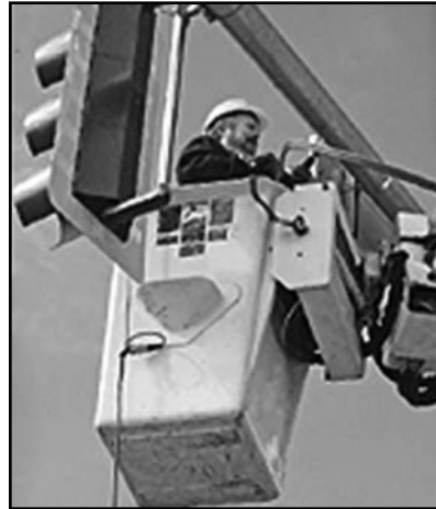
City of Victoria worker Les Keddie wires the new LED lights on Blanshard Street in front of the Save-On-Foods Memorial Centre.
