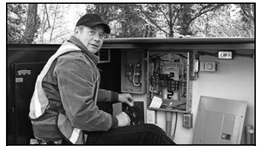
Brother D. Mackay from the City of Victoria working on a PRV station.
