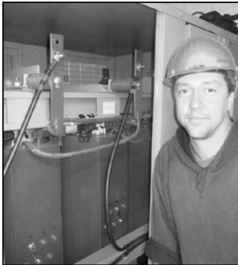
Brother Dan Stevens stands in front of the Cranes High Voltage Transformers.
