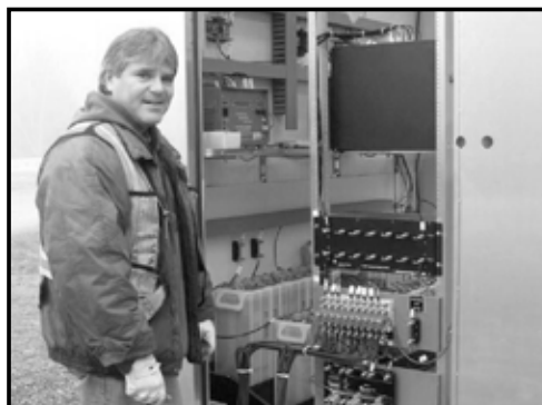
Brother Marv Bevrige from Southern Railway beside a crossing signal electrical cabinet.
