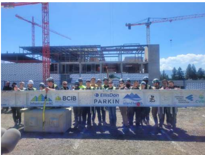
The Last Structural Beam at Cowichan Hospital with the Houle Electric Crew
