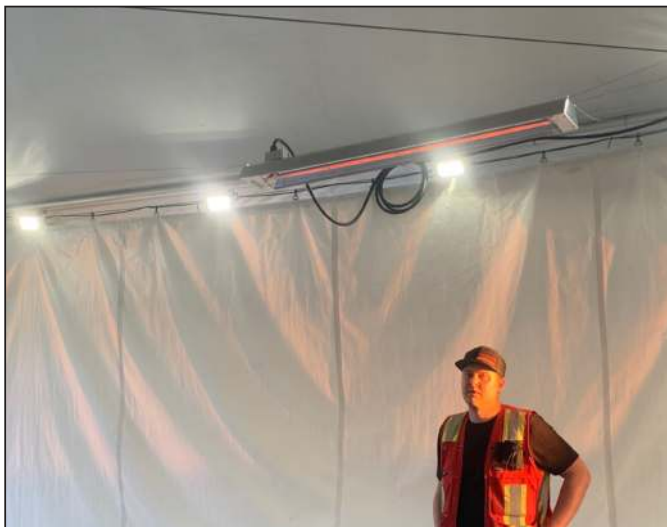
Thomis Service Electrician Mike K. wiring the lighting for Victoria COVID-19 testing centre.
